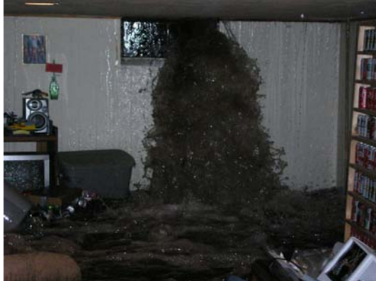
Picture showing the water pouring in.
